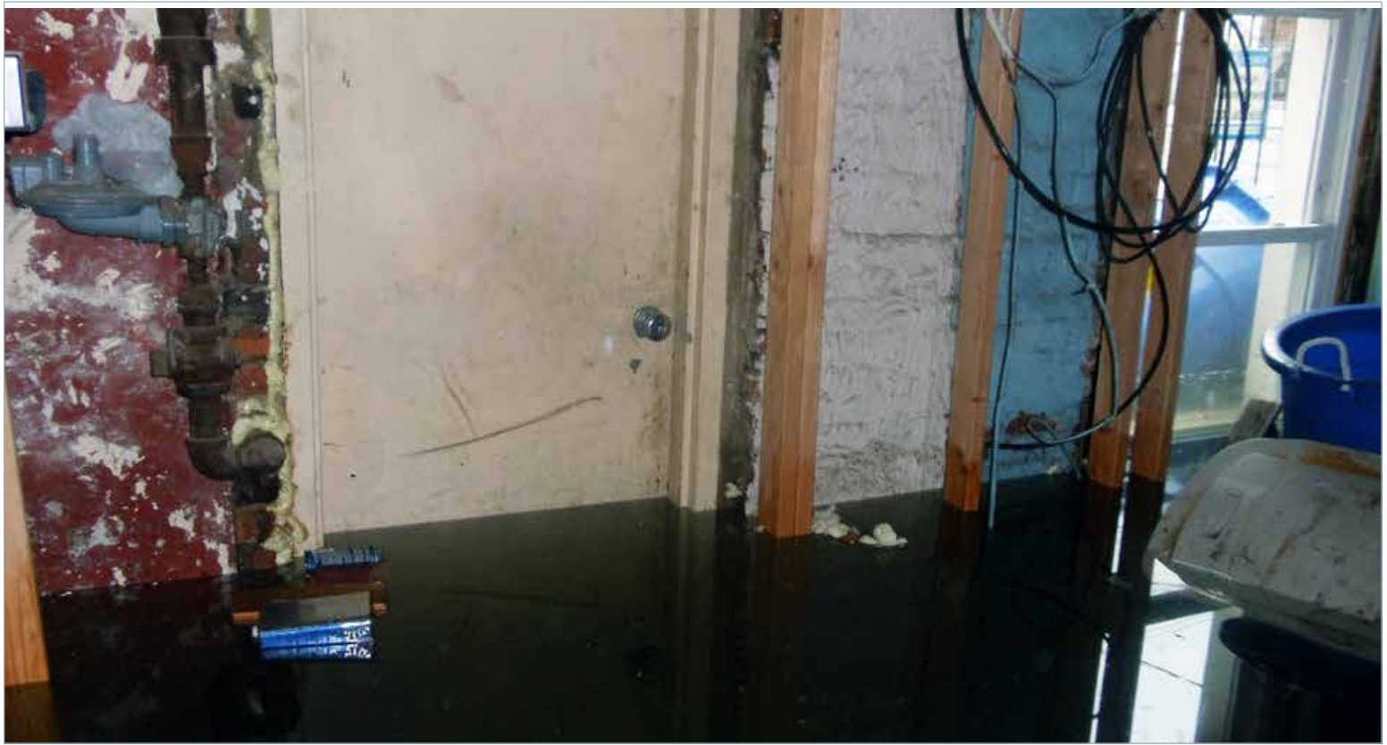
Like those of many of his neighbors, Tom Chartier's basement was hit hard by Hurricane Irene and Superstorm Sandy. While in Tom's case Hurricane Irene flooded an unfinished basement in the process of renovation (as seen in the picture), the subsequent repairs and renovations were almost completely washed away by Sandy. Photo credit: Tom Chartier.
