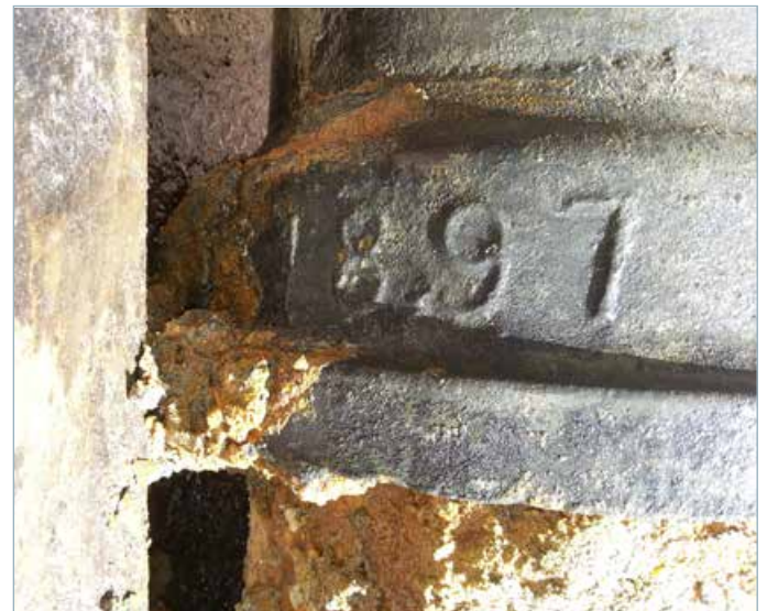
When crews repair water mains in Hoboken they record the manufacture date imprinted on the pipe and add that to their database. In addition to 1897, the dates 1857 and 1869 have been recorded. Photo credit: United Water.
