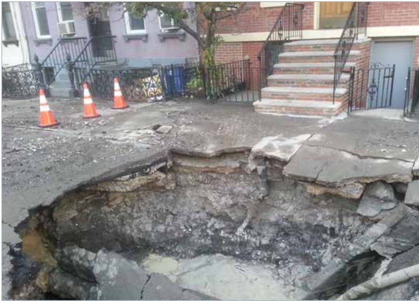
Water main breaks force the closure of roads both during (top) and after (left) the event. The stresses on a water main from a service interruption and restoration are enough to trigger additional breaks along the line.
